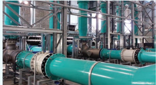
UVLX-30800-30 low pressure amalgam system operating at a UK drinking water plant
